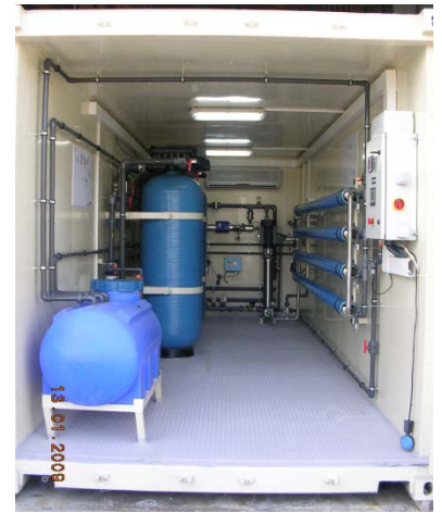
20 ft ISO containerized water treatment system – Inside View
