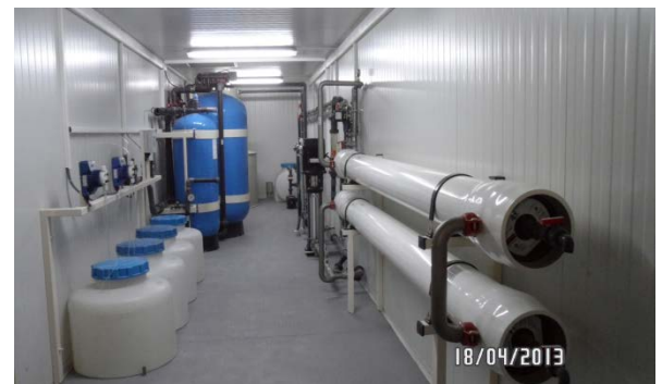
40 ft ISO containerized water treatment system – Inside View
